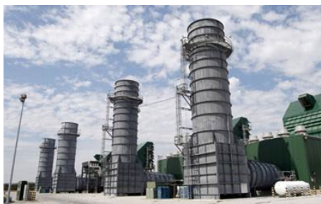
Sewell Creek Energy Facility
