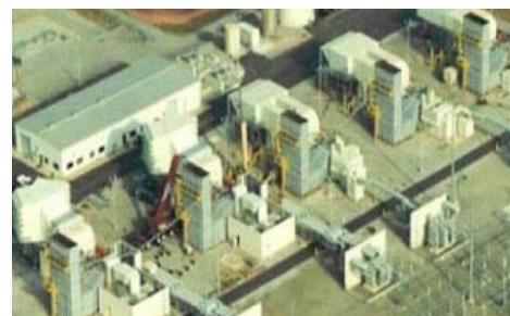
Doyle Energy Facility
